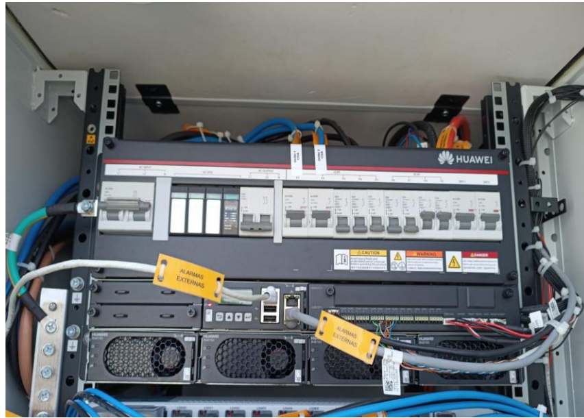
Figura 9. Power Plant HUAWEI.
