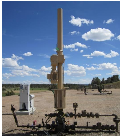
Figura 5. Sistema Linear Rod Pump instalado (UNICO, Unico's LRP Linear Rod Pump System Offers Advantages Over Traditional Pumping Units, 2015)
