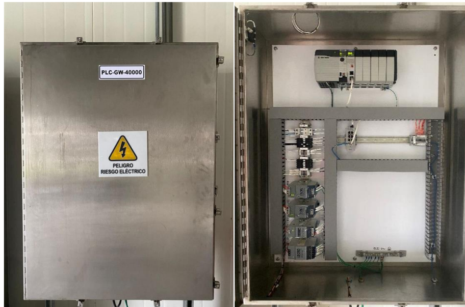
Fig. 14. Tablero de control PLC-W-40000
