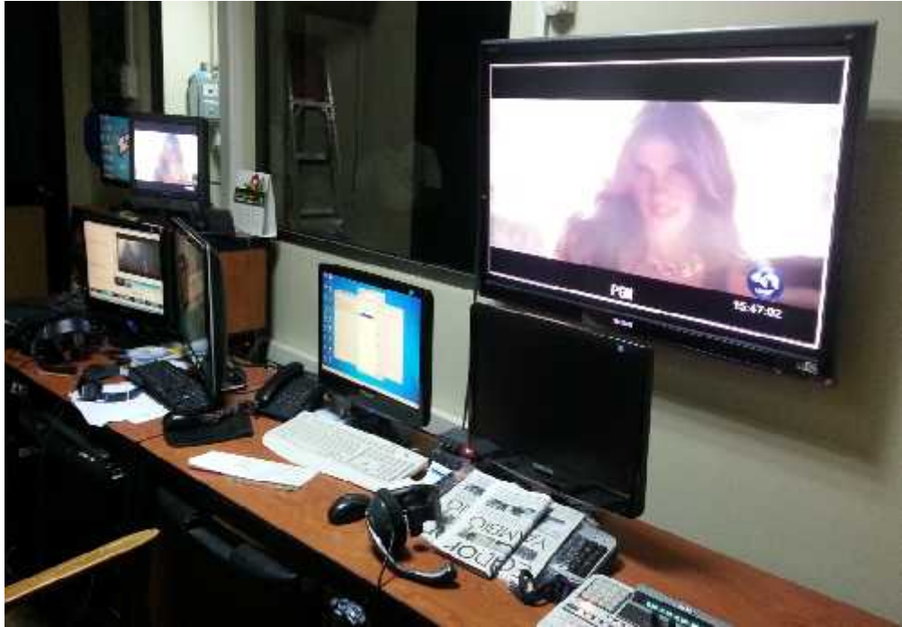
Sala Master (Switcher)
