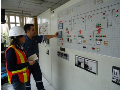
Panel de Control
